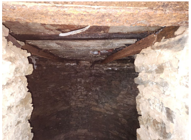
Left: Door in basement to ice house. Above: inside door is a stone lined ice storage area
