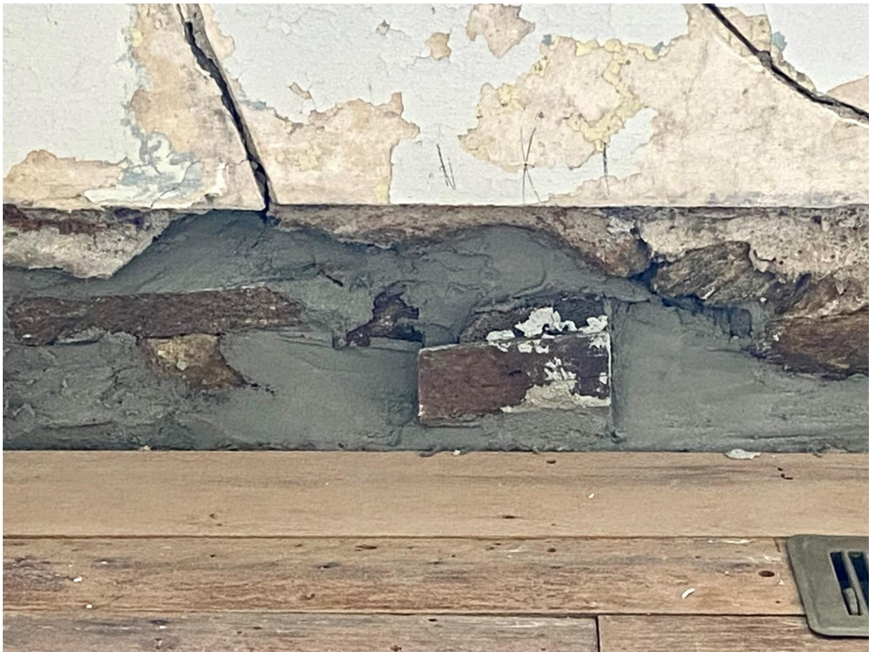
The stones were reset into the wall and gaps between were repointed with mortar. The wood mounting block for the trim was resecured.
