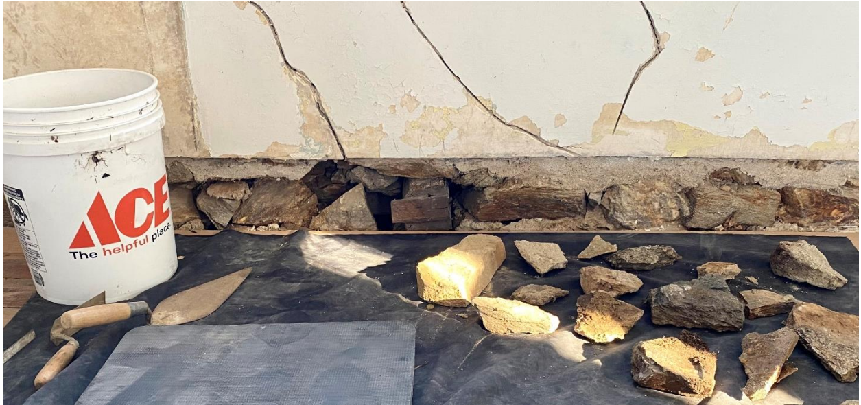
Loose stone was removed and the cavity vacuumed of dust and debris in preparation for resetting.
