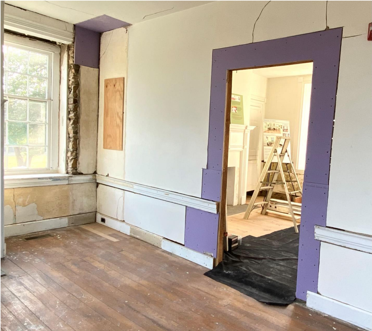
Center partition wall "AFTER". I covered the c. 1890 wallpaper panel with plywood to protect it during construction.
