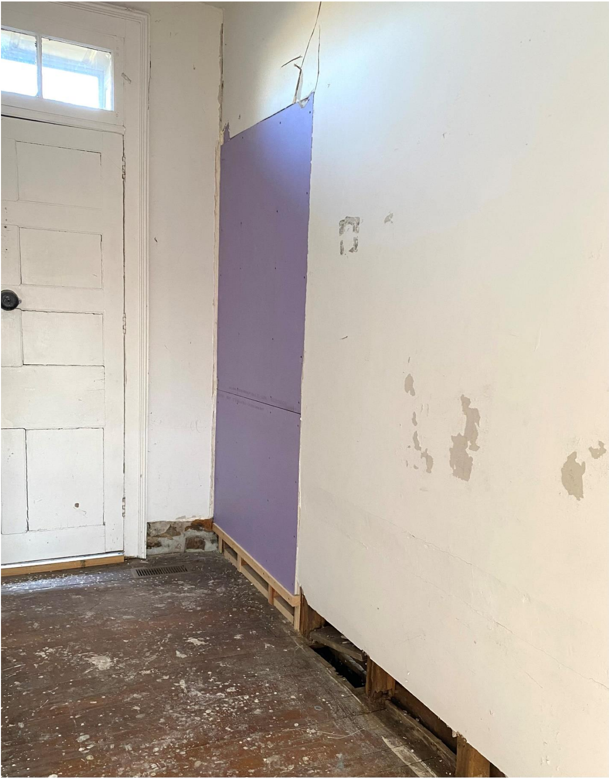
Front stair hall "AFTER". The stone wall where the baseboard was removed in the front wall was repointed.
